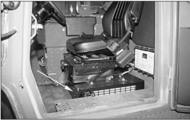
View of Air-Conditioning Unit in Cab (arrow).
