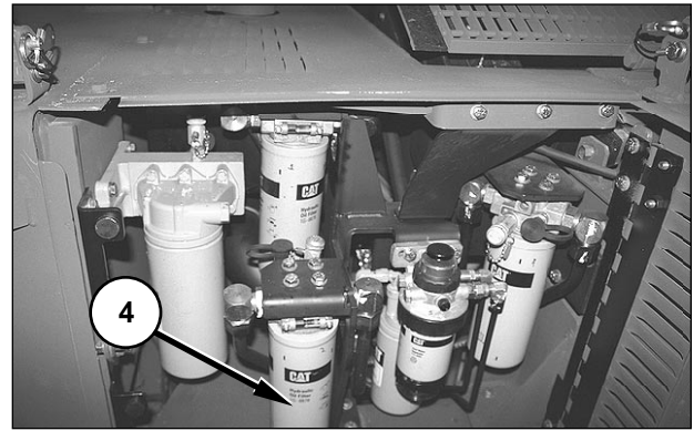
Location of Charge Filter. (4) Charge filter.
